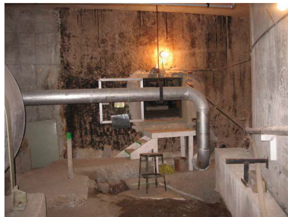
Photograph 31 N16 Tank Room
