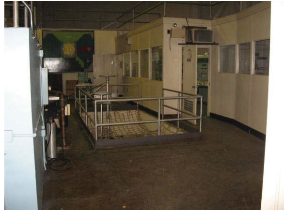
Photograph 41 Main Floor Control Deck
