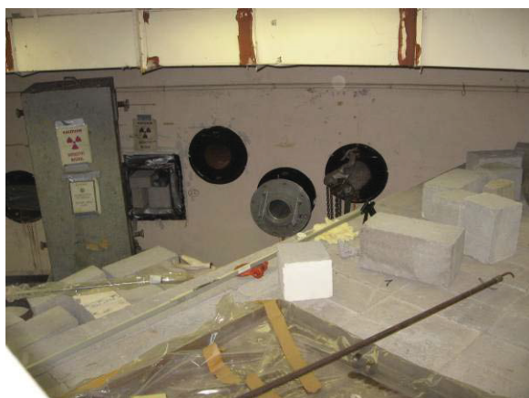
Photograph 65 Beam Port Storage Tubes
