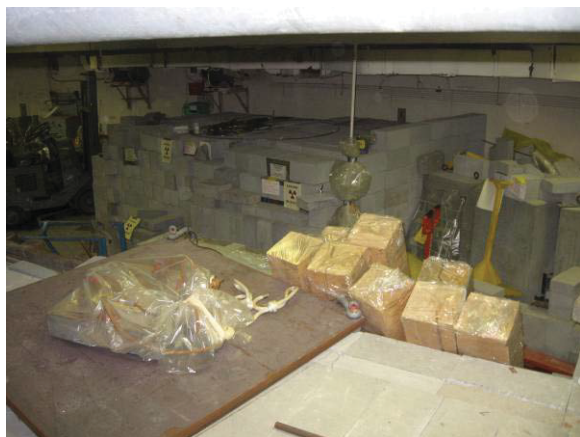
Photograph 66 High Radiation Area Neutron Level
