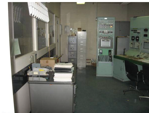
Photograph 36 Room 205 (Control Room)
