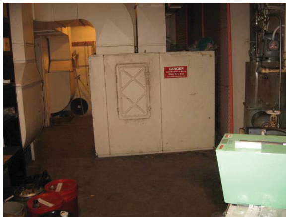
Photograph 35 Room 204 (Fan Room)
